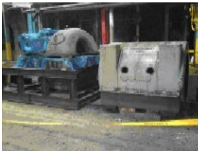
Steam Turbine & Generator
