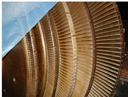
Steam Turbine Rotor
