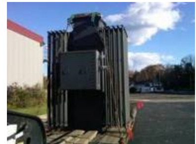
Transformer End View
