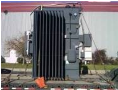
Transformer Side View
