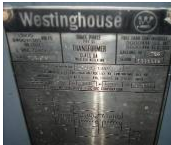
Transformer Name Plate
