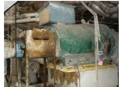
Fan Pump Motor With Cover
